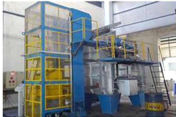
GAS-FIRED TOWER/SHAFT CENTRAL MELTING FURNACE
